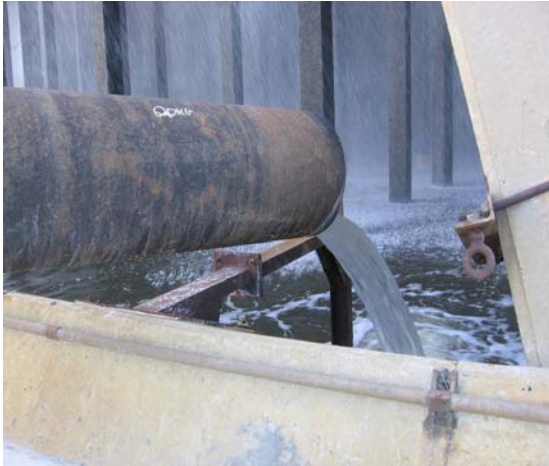
Springvale Colliery water discharging into Wallerawang Power Station cooling tower.
