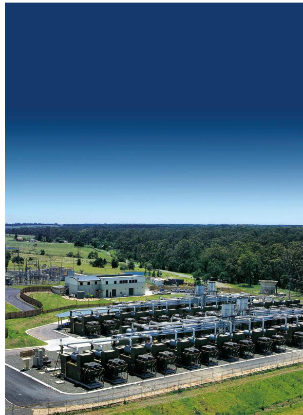
Appin Power Plant
