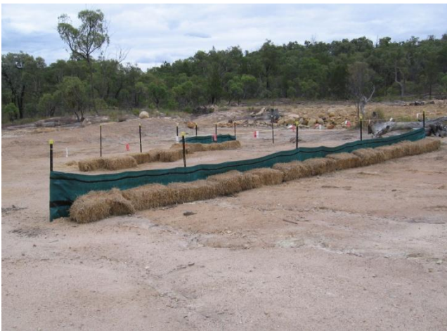
Multiple sediment fences lined with hay bales below drill site (to right of photo) in environmentally sensitive location
